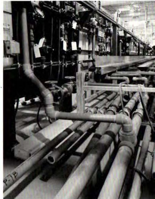
Equipment for new circuit-board plant.
