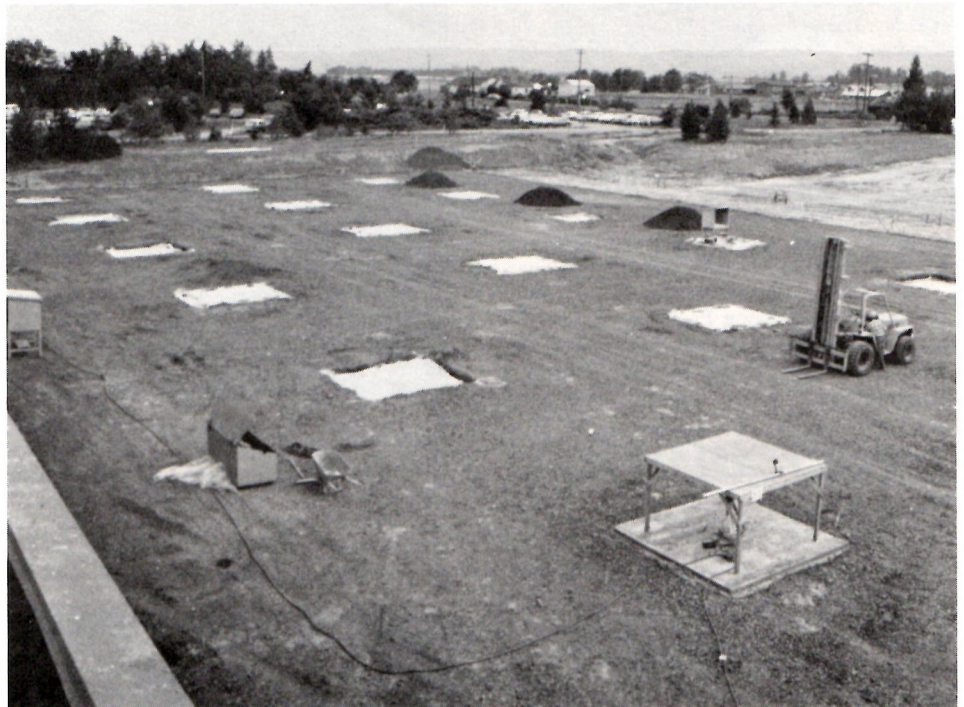
WALKER ROAD ADDITION occupies 67,000 square feet east of the present building. Photo was taken from the roof, showing concrete footings shortly after they were poured. Concrete slab floor was due to go down this week.
