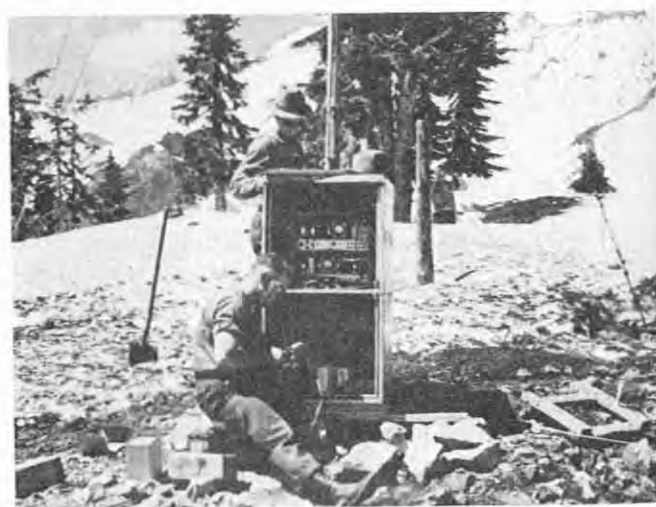
Figure 78. Logan Belleville, standing, and Carl Davis, of the Radio Laboratory, at the RRS installation on Mt. Shasta, Calif. (Forest Service photo, History Section)
