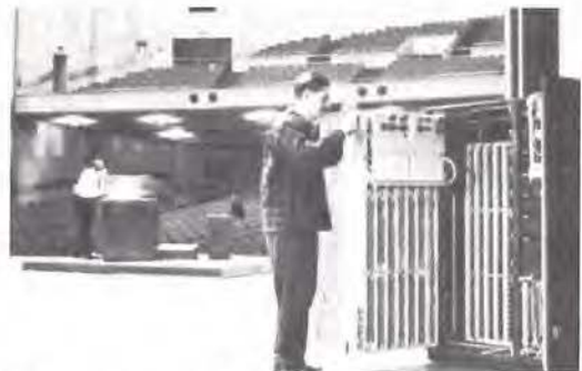
Engineers learned from the beginning that on site voicing capabilities were vital. Critical refinements on all Rodgers Organs are made during the installation in order to best tailor the scaling of the organ to its particular individual acoustical environment.
