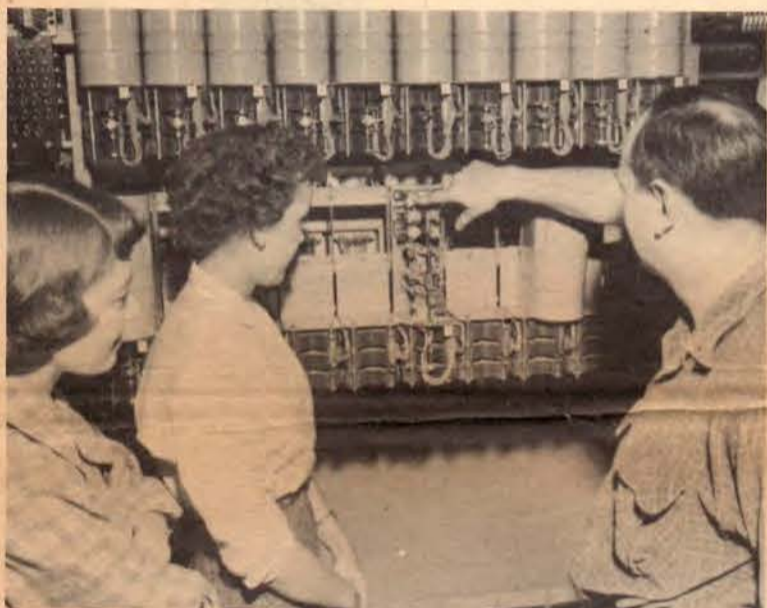
Bob Herren explains to Maryellen Stevens and Hallie Todd the intricacies of the new switchboard operation which is now in effect at Tektronix. Number please!
